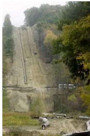
Work on the Millennium Pipeline project as seen from Route 26 in Union Center in 2008. (File photo)
