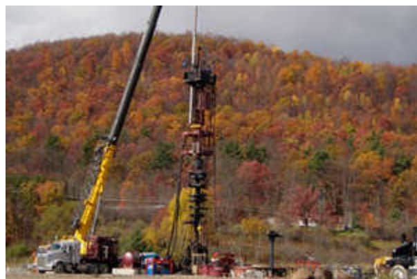
Workers adjust a drilling rig at Anschutz Exploration Corp.'s natural gas well in Big Flats, N.Y. (Peter Mantius/ DCBureau.org )
